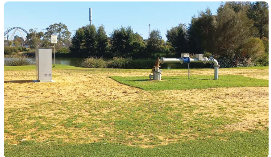
Completed Bore 2A. The electrical cabinet (left) houses the control system where the performance of the bore is measured.
