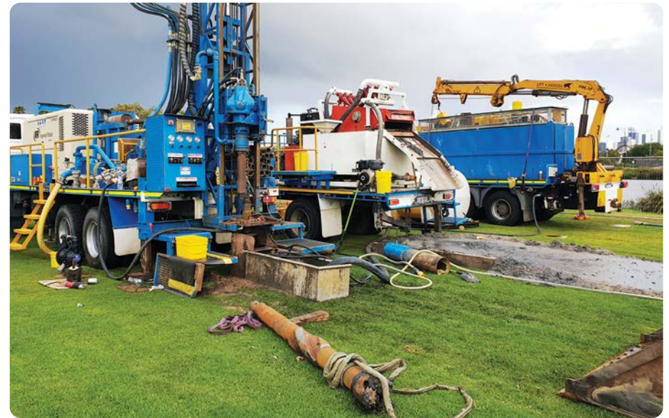
Bore 2A under construction use a Mud Rotary drilling rig. The large cutting tool at the base of the machinery is used to cut through the soil profile to reach the required depth.
